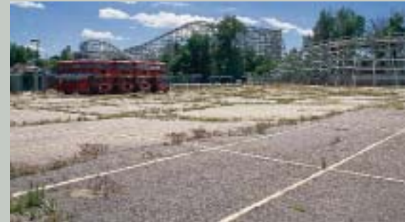
Debris from the demolition of the old Elitch Gardens amusement park was recycled.
