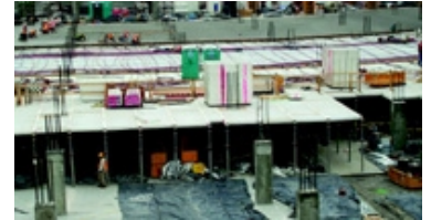
On this congested inner-city site, workers are building the first below-ground parking garage level. In the background one-third of the deck is being finished while deck forms are being positioned for the middle third. Photo: Hensel Phelps
